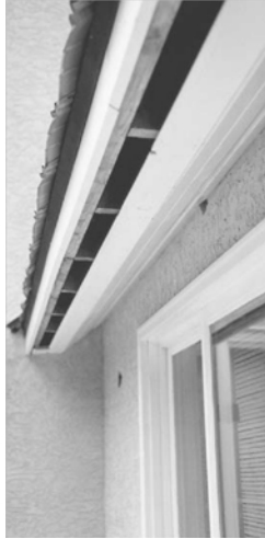
Vents not screened
